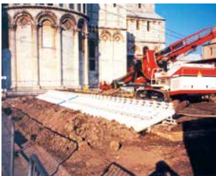
Drainage was part of the solution to stabilising the Leaning Tower of Pisa
